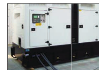
Enclosed power outlet, terminal and sockets
