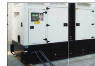
Enclosed power outlet, terminal and sockets
