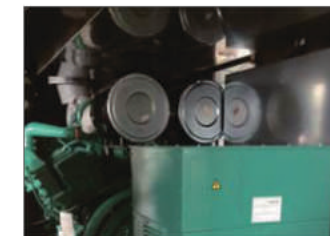
Interior of the genset
